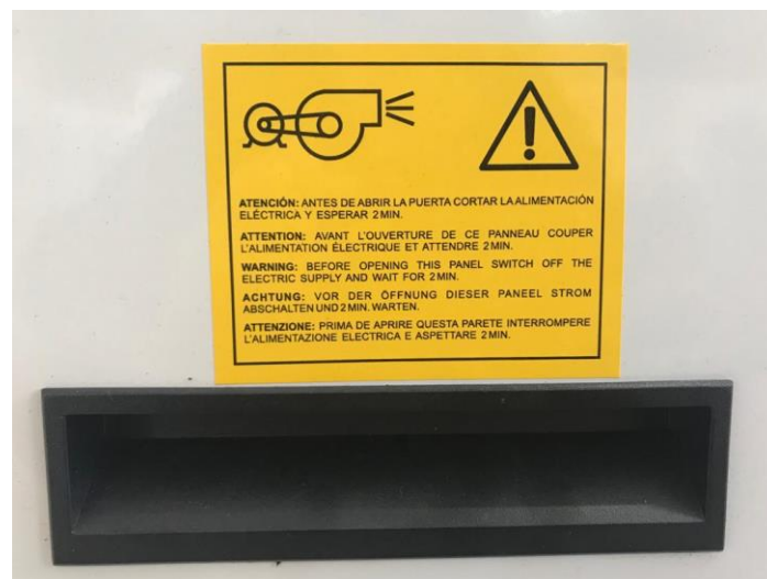
Safety labels on the unit
