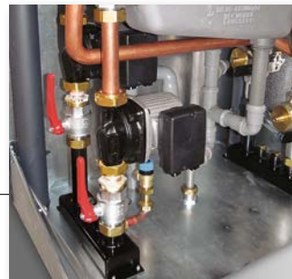
Pumps and gate valves
